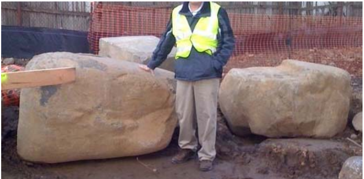
Figure 9 – Boulders Removed in the Upper 25-ft of Queens NY Site to Facilitate ACIP Pile Installation
